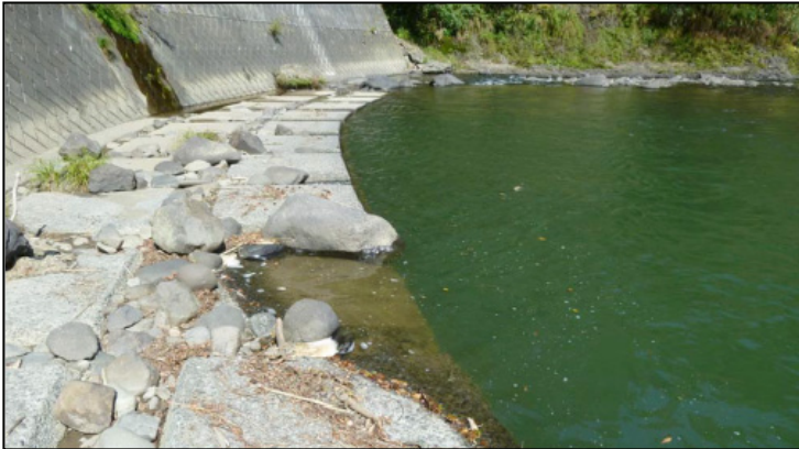
This photo shows a typical concrete bulkhead on a river cut bank. During flooding the structure may not sustain visible damage, but the base and fill area behind bulkhead may scour and weaken the entire structure and potentially destabilize the area.
